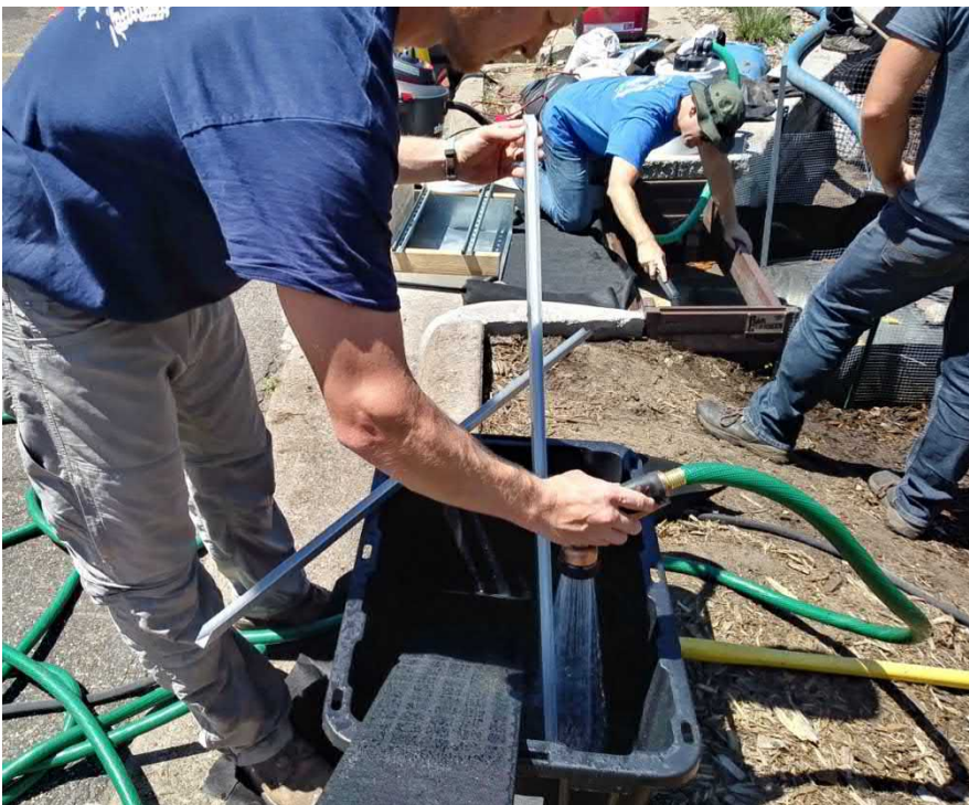
Figure 36. Rinsing the partially disassembled Rain Guardian Bunker screen wall in a bin (foreground) and vacuuming captured sediment from the bunker (background).
