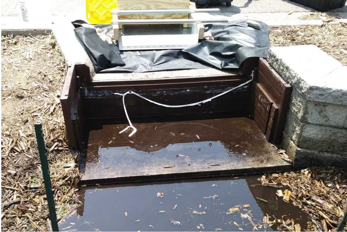
Figure 4. At the Anoka site, the outer frame and concrete pad of the Rain Guardian Bunker device was left in place and adapted for all tests.
