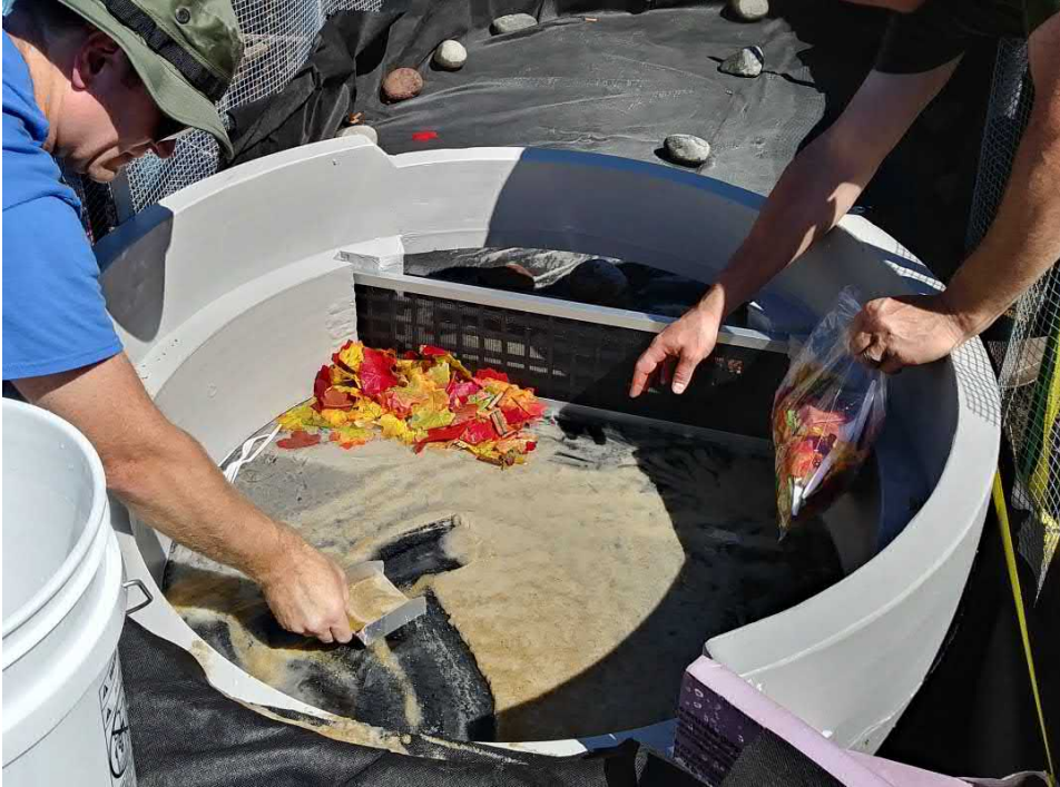
Figure 40. Cleanout gross solids and sediment from the Rain Guardian Turret.
