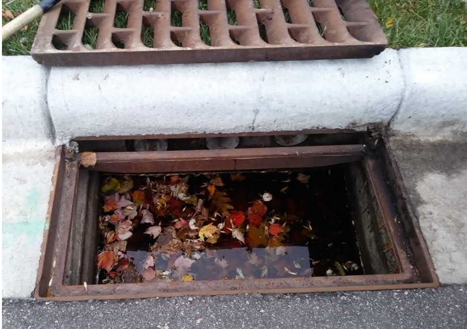
Figure 13. Shallow sump pretreatment with surface grate removed. This photo was taken upon arrival at the site, before cleaning the sump in preparation for testing.
