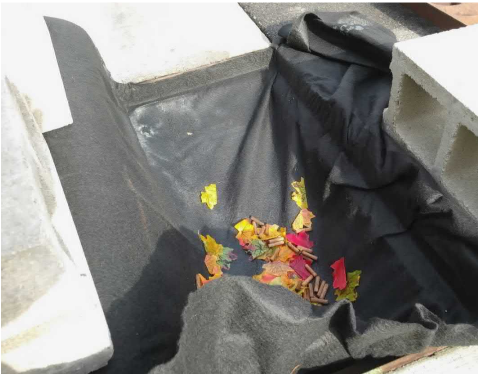
Figure 50. Gross solids and slight amount of sediment captured on geotextile fabric in the downstream catch basin frame (BBP-012-A).
