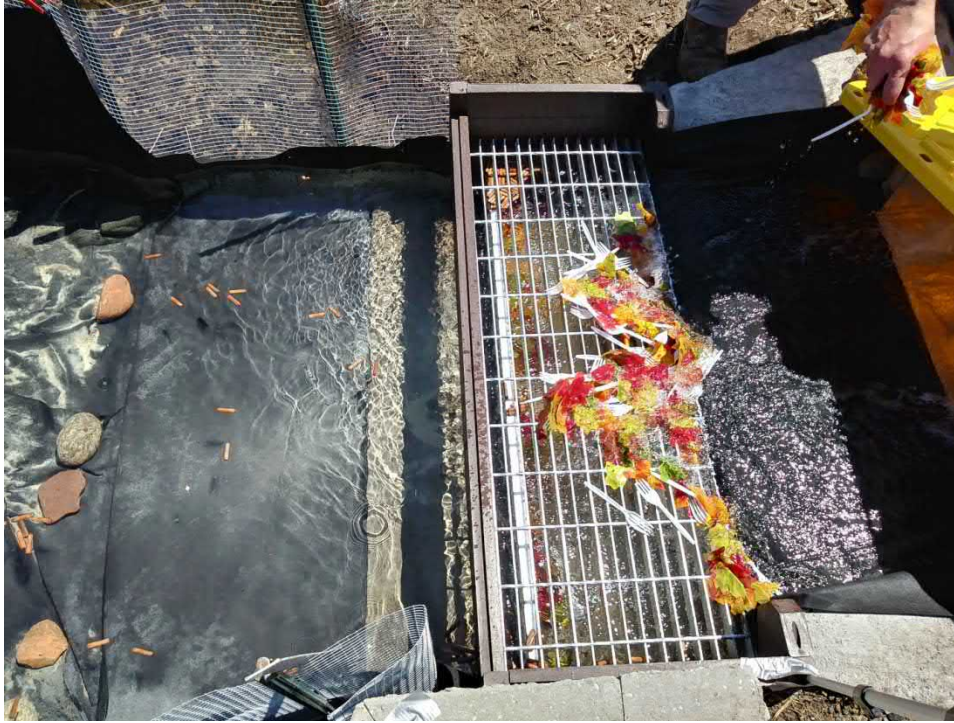
Figure 8. Overhead view of Rain Guardian Bunker (RGB) at 0.25 cfs during gross solids addition (RGB-025-B). Entrance from the curb cut comes into the RGB from the right of the picture; flow through the screen wall exiting the RGB in the center of the picture towards the left.
