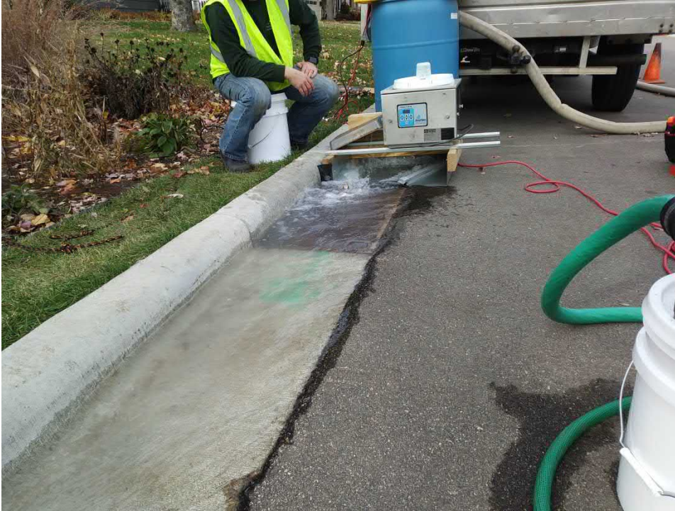
Figure 49. Flow in the gutter during bypass (BBP-025-A).
