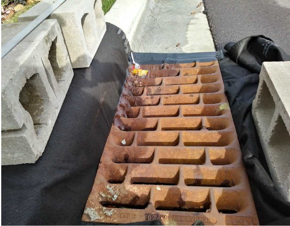
Figure 48. For the bypass tests of the Bloomington pretreatment practice, the downstream catchbasin was lined with a geotextile basket to capture sediment and gross solids bypassing and/or washing out of the pretreatment practice.
